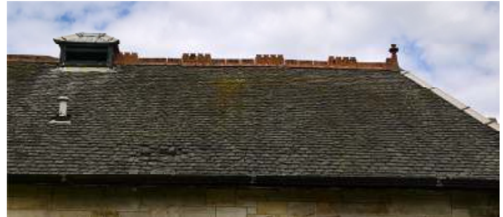
Slates missing and slipped
