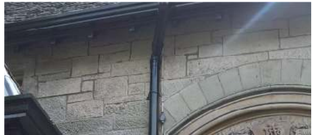
PVC downpipes in use
