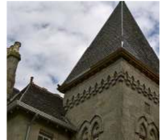
Roof flashing missing - Spanish slates in use
