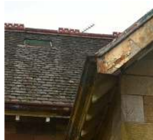
Blocked and corroded guttering
